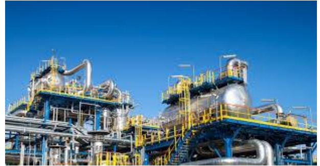
Figure 24 A Sulphur recovery unit in China.
